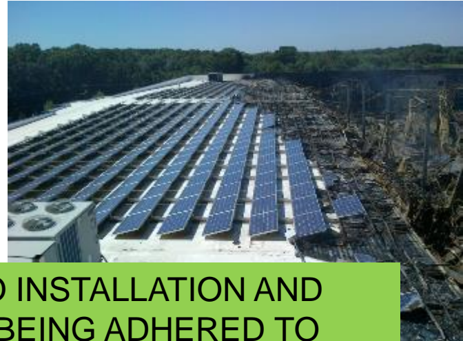
Combustible root insulation
